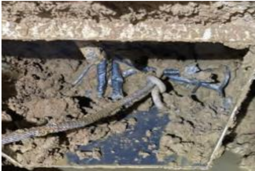
Fig. 8. Difficulty in discharging slag
